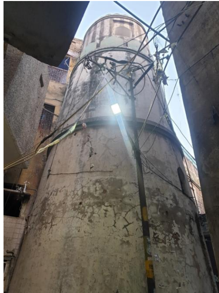
Fig. 12: Deterioration of the structure.
